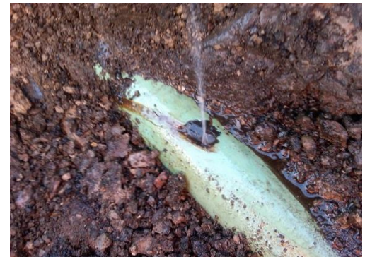
Active leak in Chadron
