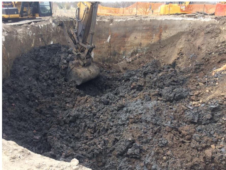
Excavation of contaminated soil impacted by coal tar waste in the below grade gas holder at the FMGP site in Beatrice.
