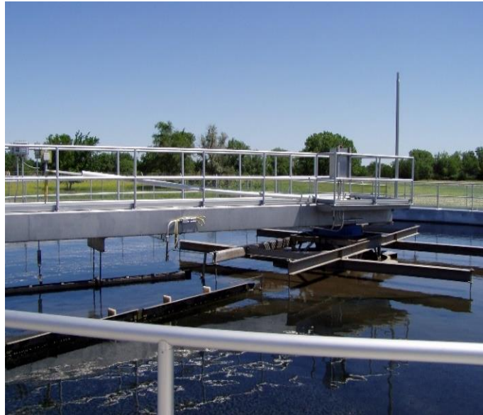
This photo shows a Wastewater Treatment Facility for Lincoln.
