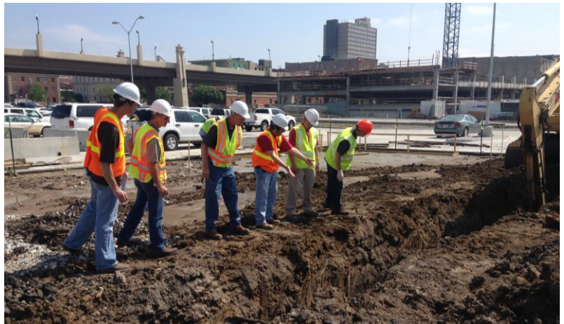
Staff observe remediation at the West Haymarket Voluntary Cleanup Program site in Lincoln. See page 35 for more information on the Voluntary Cleanup Program.
