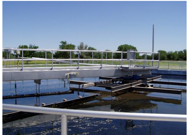
This photo shows a Wastewater Treatment Facility for Lincoln.
