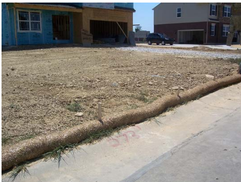
Make sure filter log stakes are spaced to prevent undercutting or bypasses. Leave stake tops extended along sections to prevent drive-overs. Photo credit: Barry Tanning, Tetra Tech
