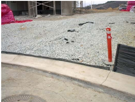
Good application of rock exit pad. Note short section of material against curb that is keeping rock from leaving site. Photo credit: John Kosco, Tetra Tech.
