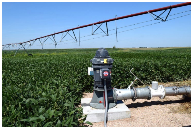
New electric motor in place at center pivot.
